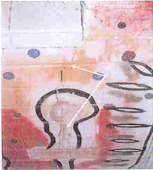
Visible cracks in Brickwork outside the building.
