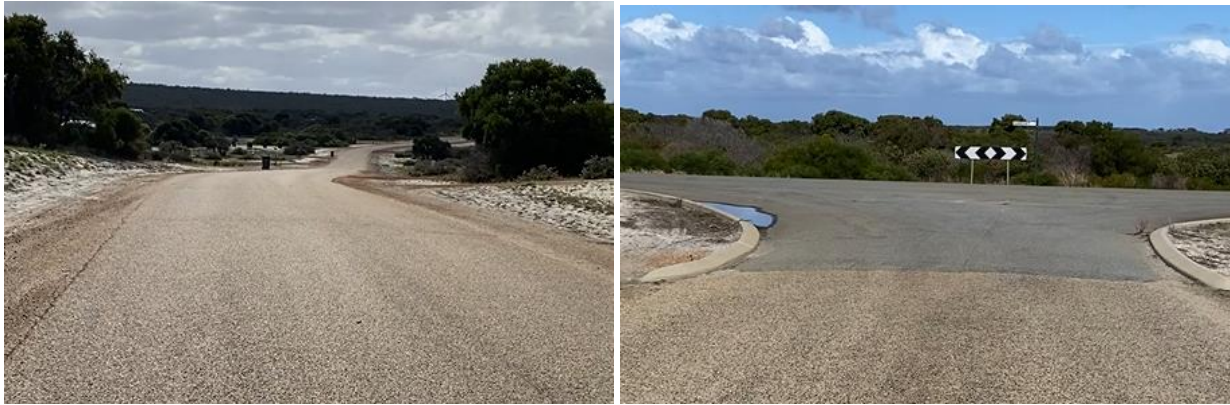
Figure 4-37: Boroonia Street from Banksia Road
